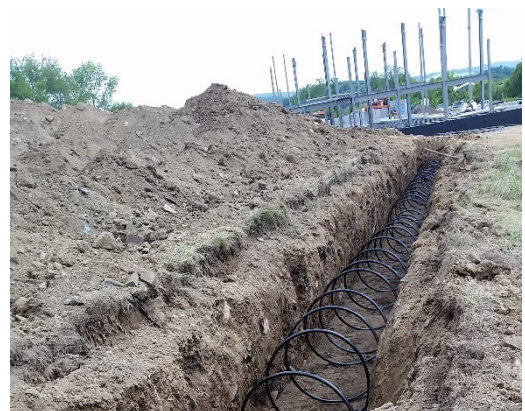
Ground Source Heat Exchanger at PS21: Performance Spaces for the 21 st Century
